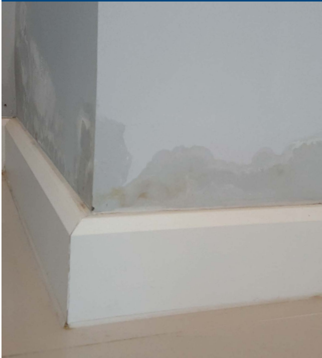
Visible rising dampness in internal walls
