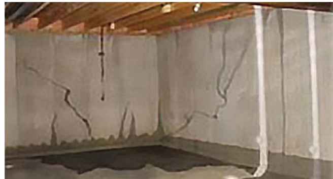
Difficult to trace the source of leakage
