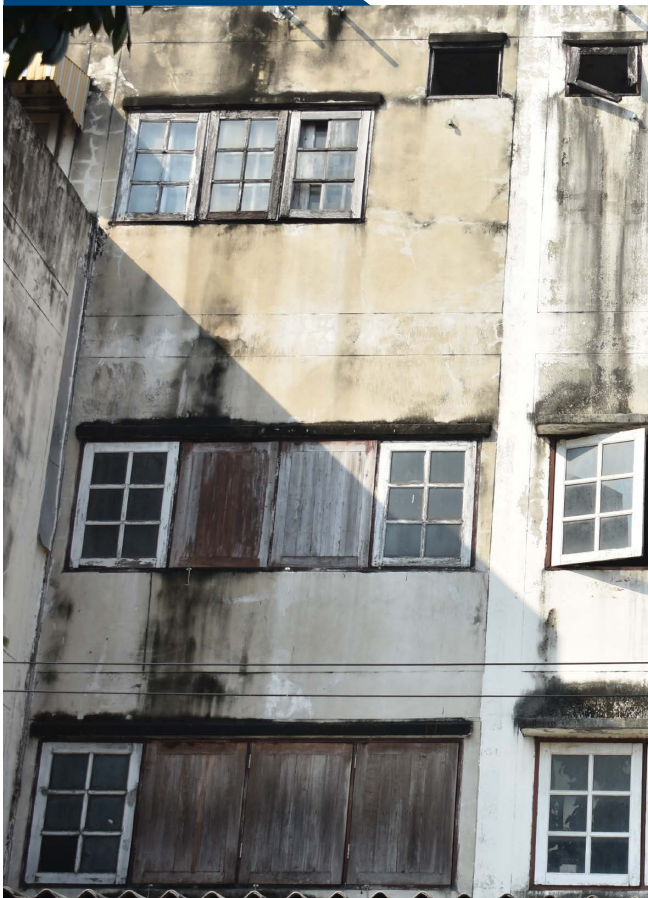
Dull Exterior Walls
