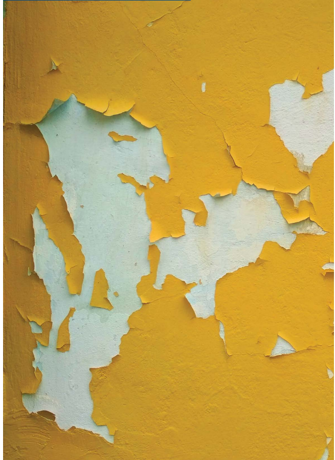
Paint Peeling Off
