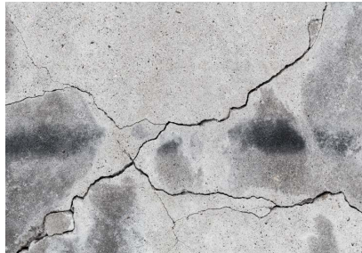
Plastic shrinkage cracks
