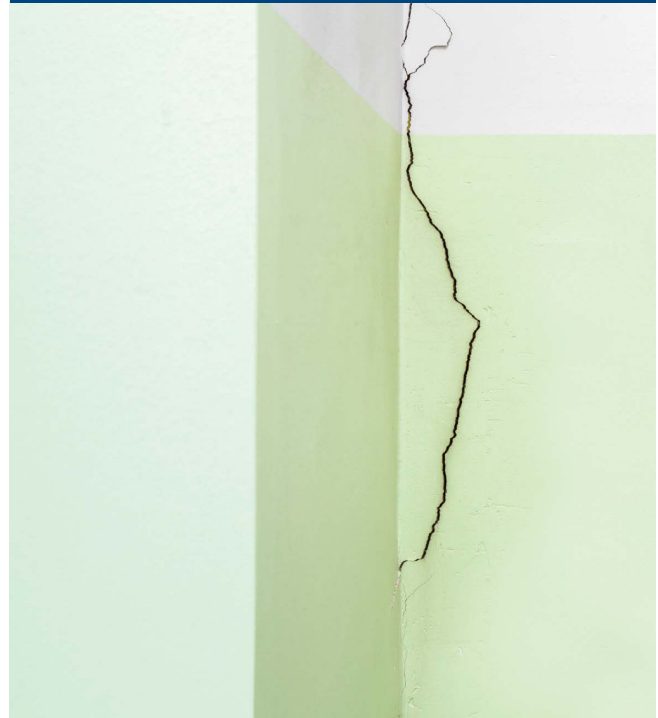
Crack formation on walls
