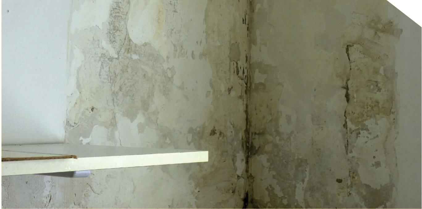
Peeling paint from dampness/seepage from adjacent wet areas (bathroom, balcony, kitchen)
