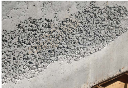
Honey combing due to Improper compaction
