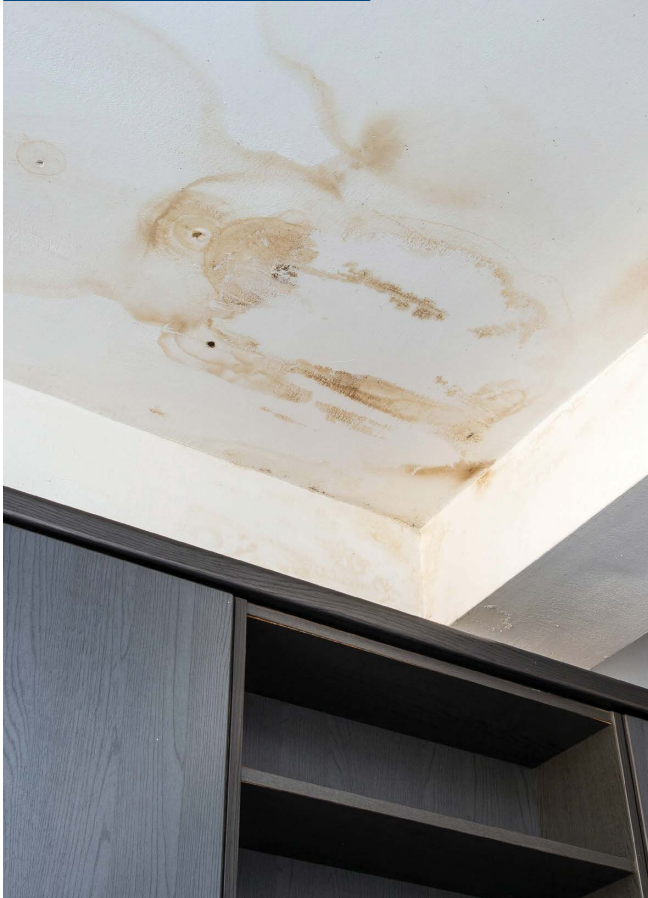
Damp Ceiling & Walls
